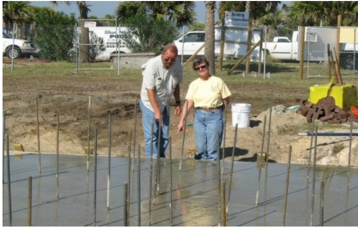
Dennis Barnell and Terry Kemp left a gold dollar coin in the finished concrete base. Dennis had tossed an additional coin deep into the foundation as the first load of concrete was poured.
