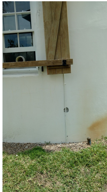
Lightning traveled down and out the bottom of both sides of the lighthouse
